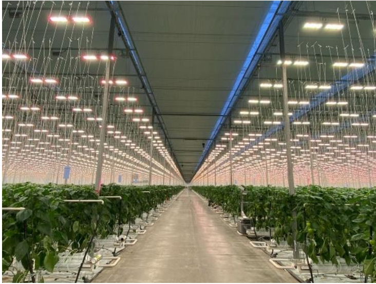
Powering of the greenhouse sector with DER solutions
