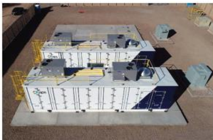
Exhibit 139 – BESS commissioned by Arizona Public Service [83]
