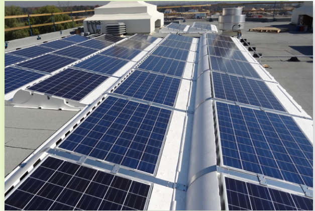
Over 4,300 MW of distributed energy resources are in service and under development in Ontario, including the 10kW project built on top of the Devi Mandir Hindu Temple (pictured).
