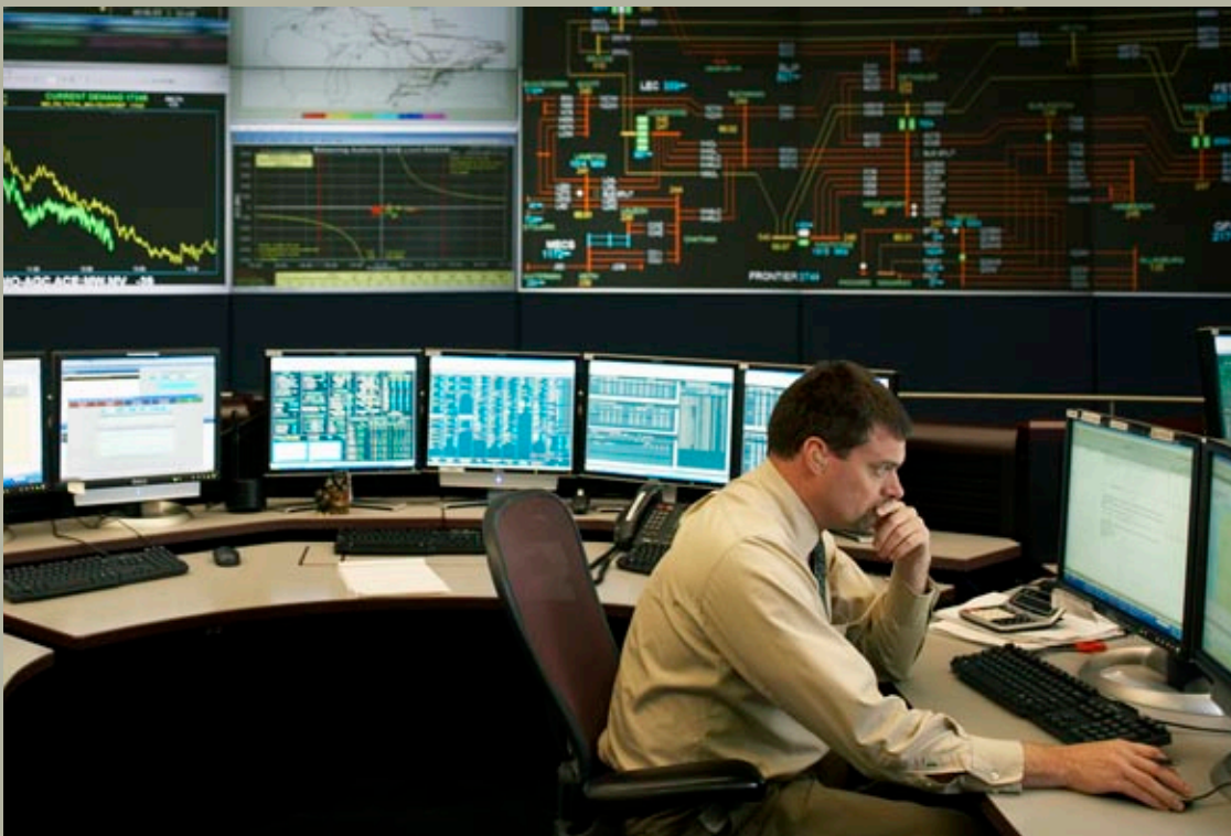
IESO Control Room
