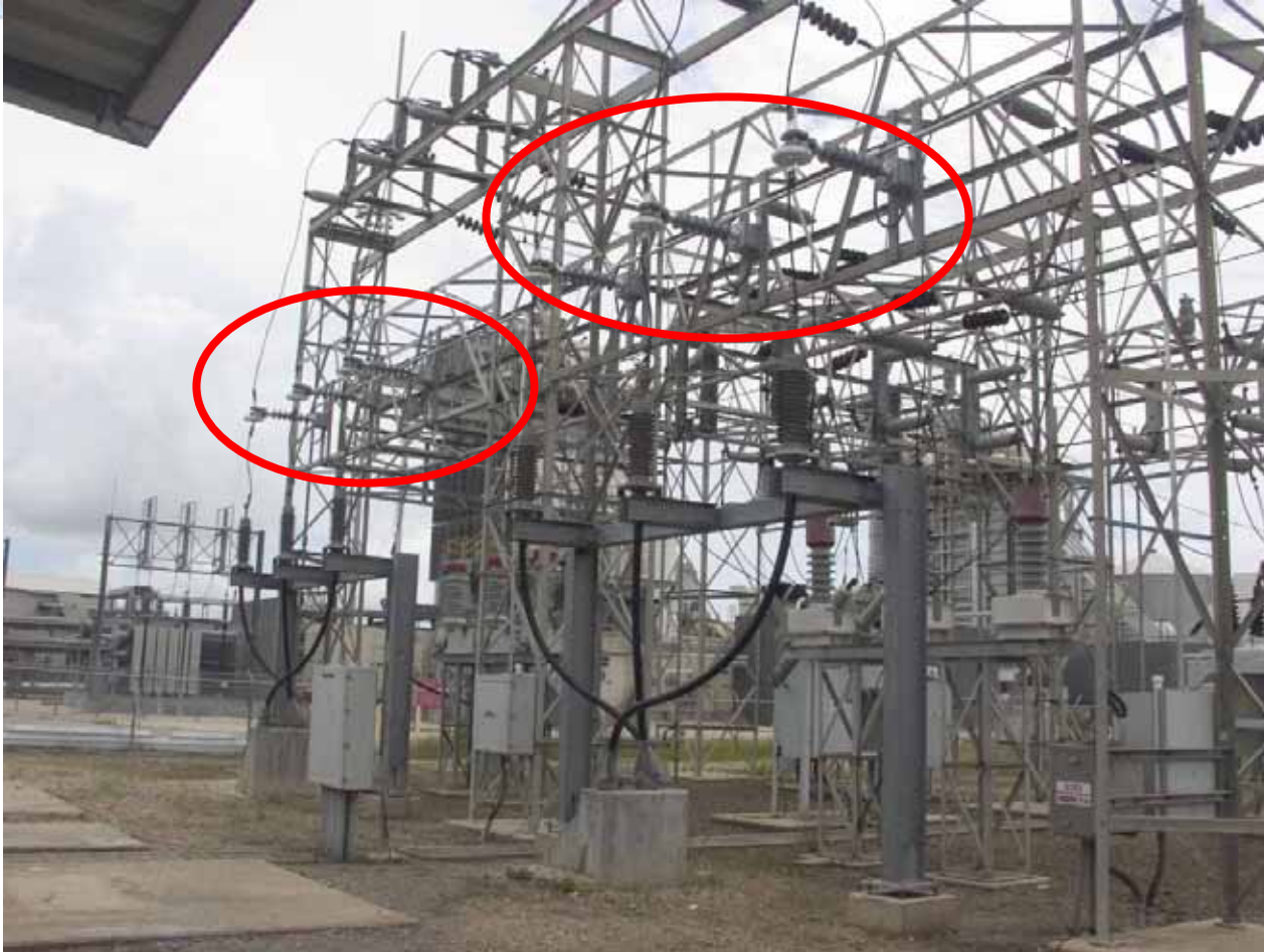
Entergy Gulfrich Substation – 69 kV Optical Current Sensor
