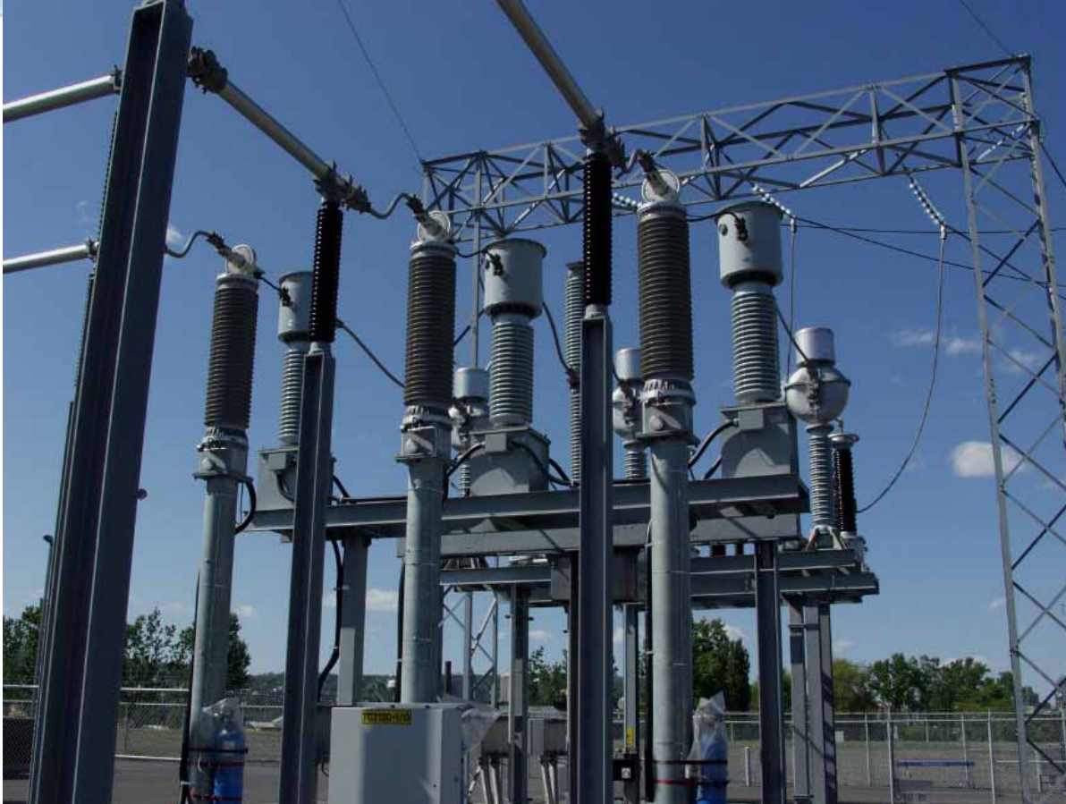
Hydro Quebec's Rolls-Royce Substation – 115kV Combined Voltage & Current Optical Sensor
