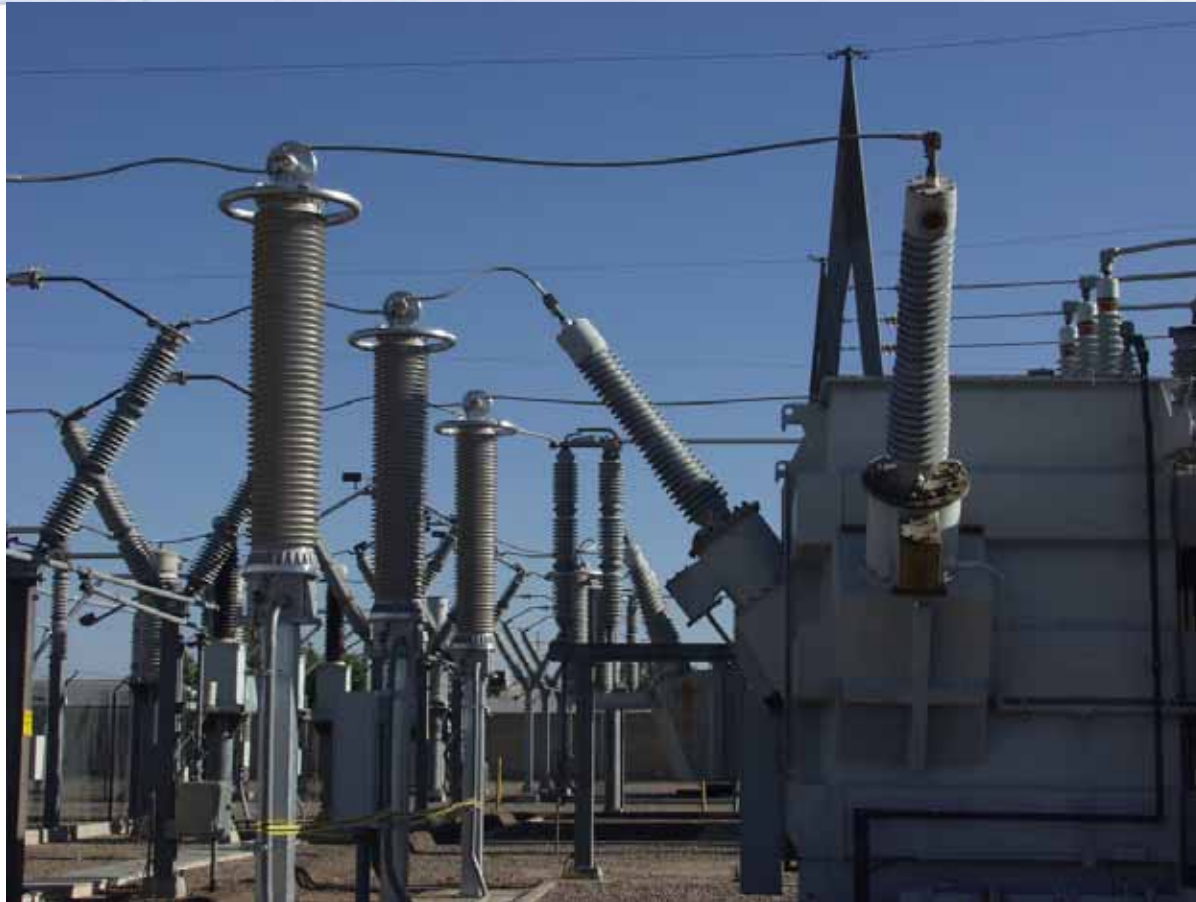
APS's Deer Valley Substation – 230 kV Combined Voltage & Current Optical Sensor
