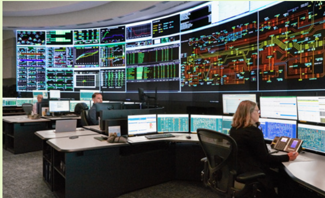
The IESO control room oversees the provincial power system and market in real-time.
