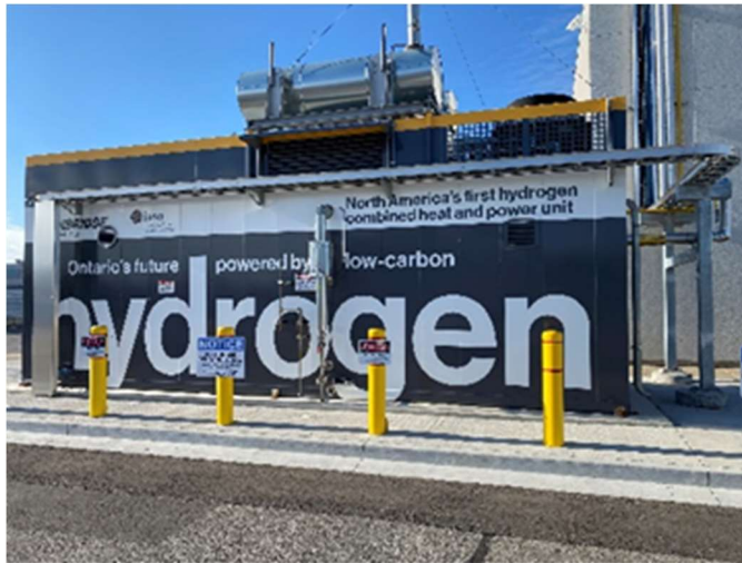
Installed system in fully operational state.
