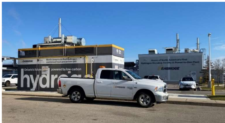
Installed system in fully operational state
