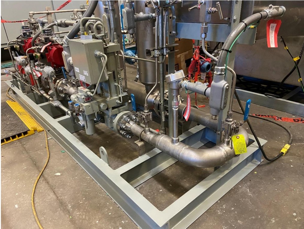
Fig 6b: H2 blending skid – manufactured for a similar project
